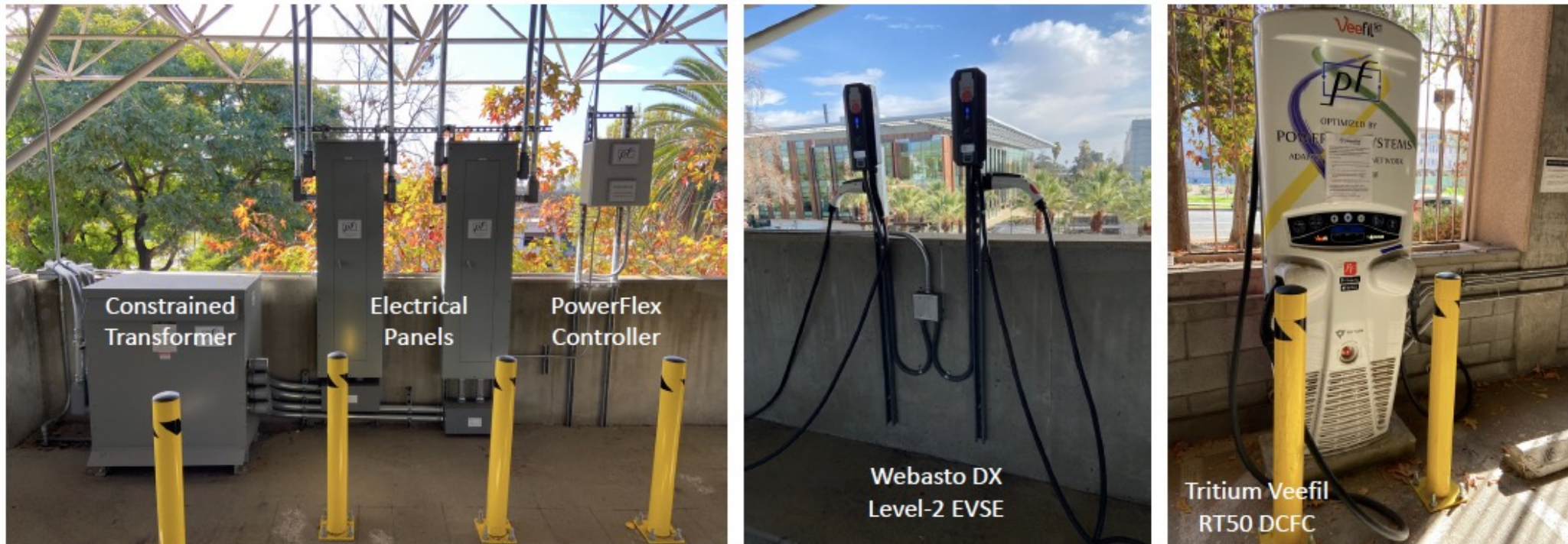
Figure 1. Photos of the N_Wilson_Garage_01 ACN, which is one of the charging sites used to collect data.
