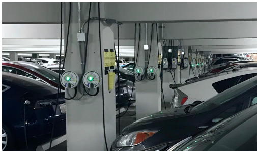
Fig. 1. Photograph of the ACN testbed.
